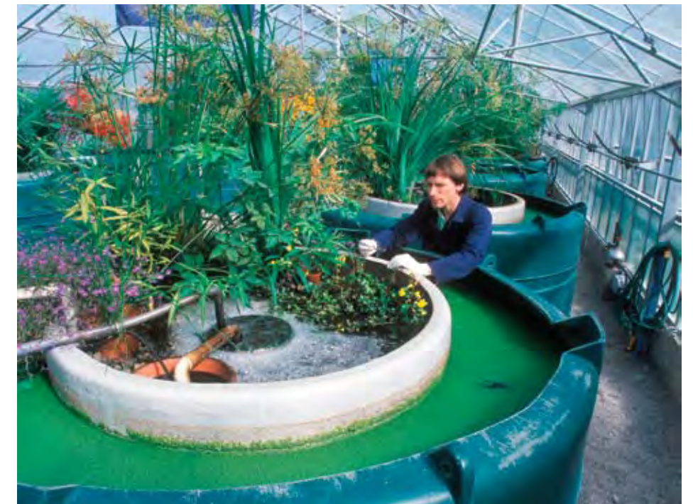
IN THE SCOTTISH ECOVILLAGE FINDHORN, THE COMMUNITY'S WASTEWATER IS PURIFIED THROUGH A TREATMENT PROCESS THAT INVOLVES VARIOUS TANKS.
